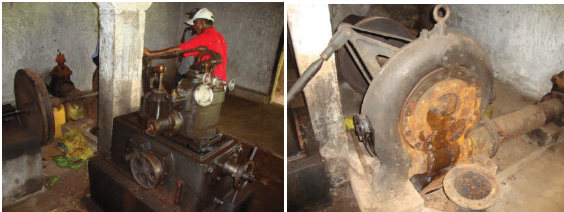
Turbine and other equipment at the hydro power plant
